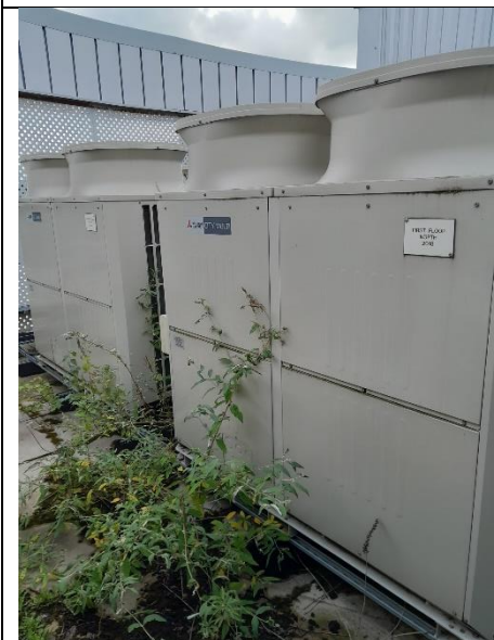
Chiller external (perimeter enclosed) roof area
