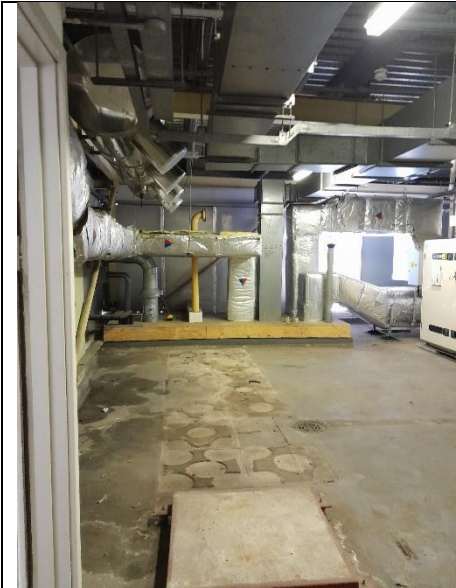
Internal plant room
