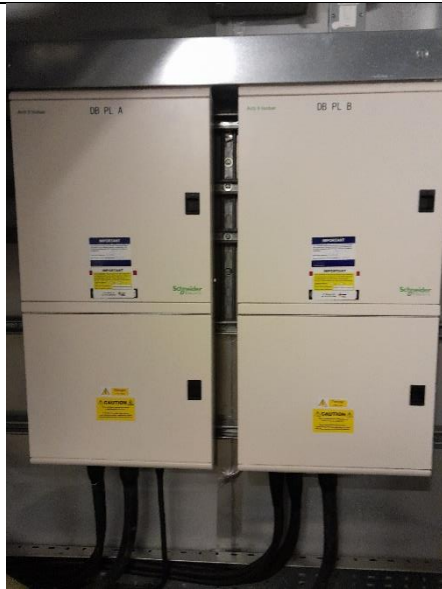
Plant room electrical
