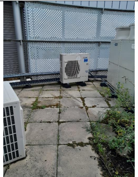
Chiller external (perimeter enclosed) roof area
